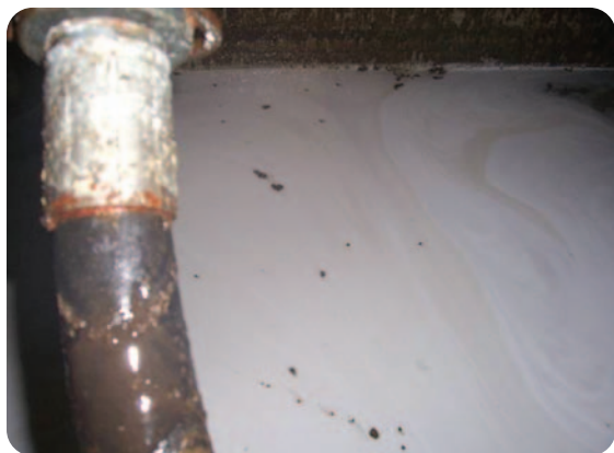
Before using QUINTOLUBRIC® in the longwall tank.
